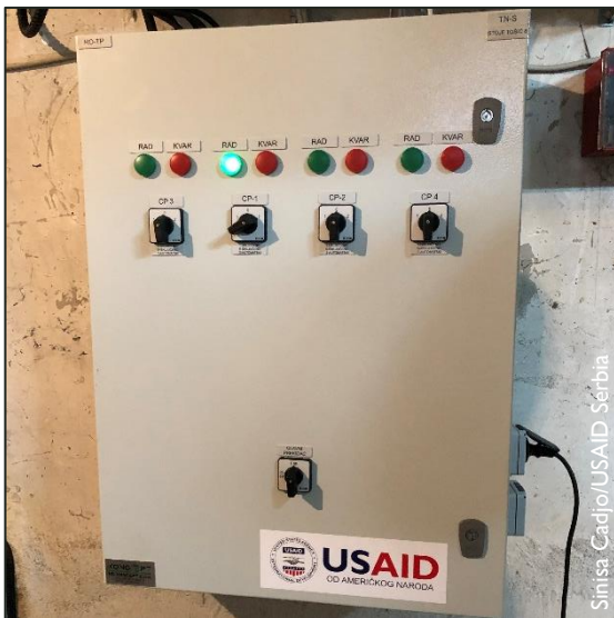
JKP Čačak SCADA Control Panel
