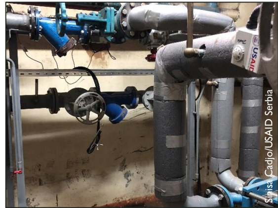
JKP Čačak SCADA Temperature Sensors
