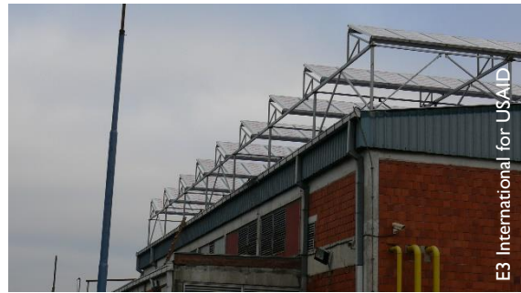
The JKP Grejanje roof-mounted solar thermal system on the Kotež boiler house.
