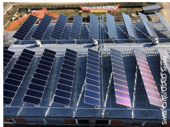
The JKP Grejanje roof-mounted solar thermal system on the Kotež boiler house.
